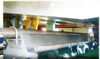
02 Belt Washing Nozzle (Shower Box)
